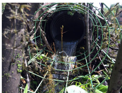
Another section of pipe carries water from the dam, emptying
