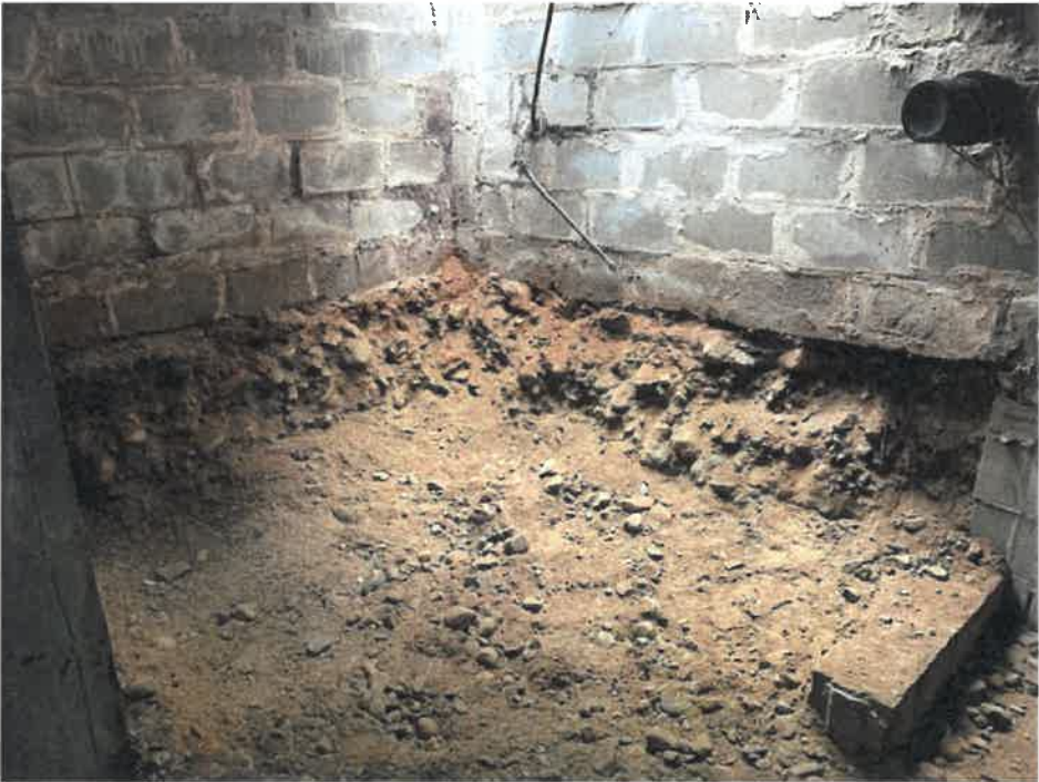
Photo of foundation once depth was verified during excavation of existing crawl space.
